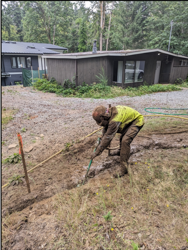
Photograph 1. Connor McDermott, of Tree Solutions Inc, Using an AirSpade to open a trench at the proposed limits of excavation.
