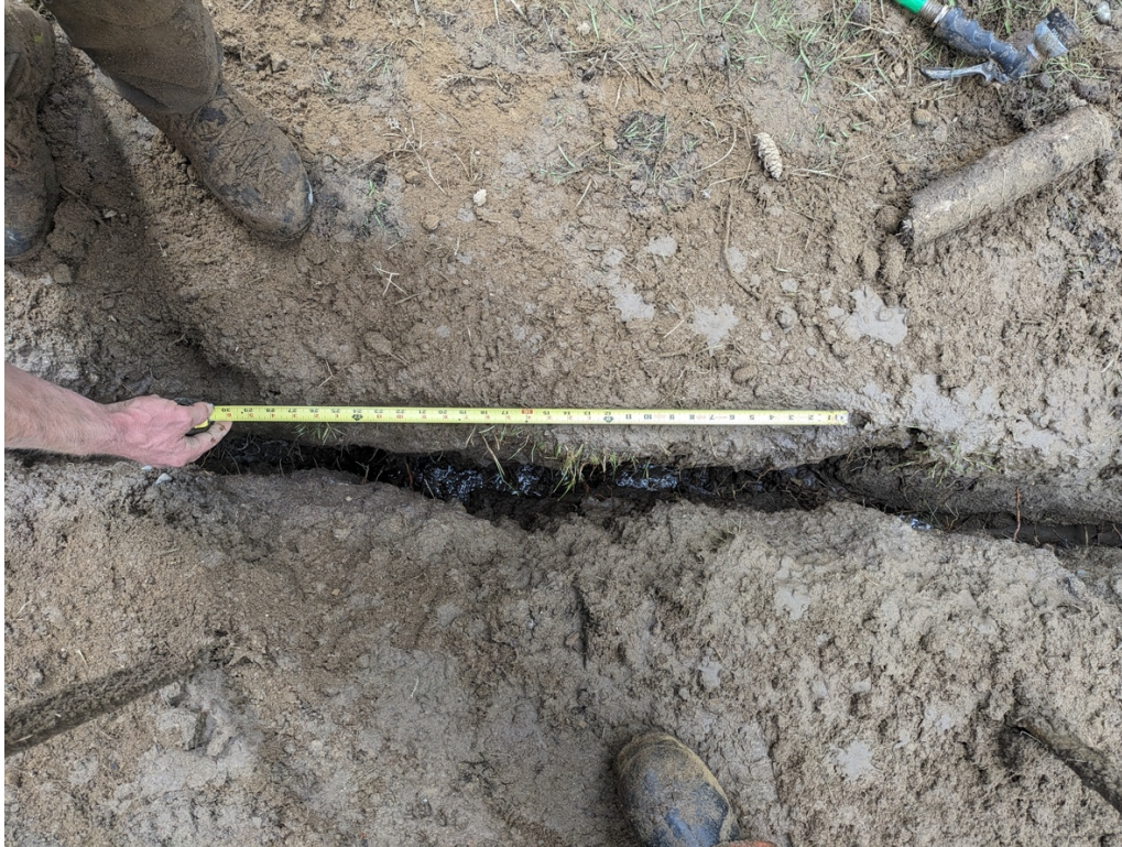
Photograph 4. A typical section of trench. Small feeder roots can be seen at right.
