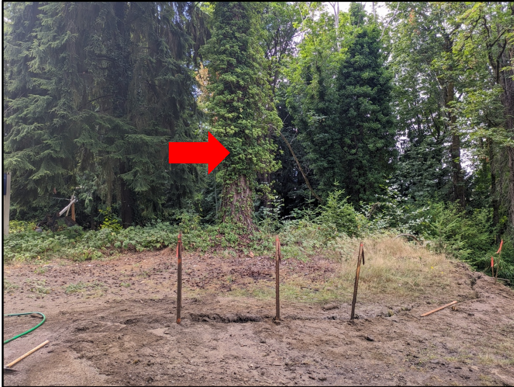
Photograph 2. Our completed trench as marked by stakes and flagging. Tree 1005 is indicated with a red arrow.
